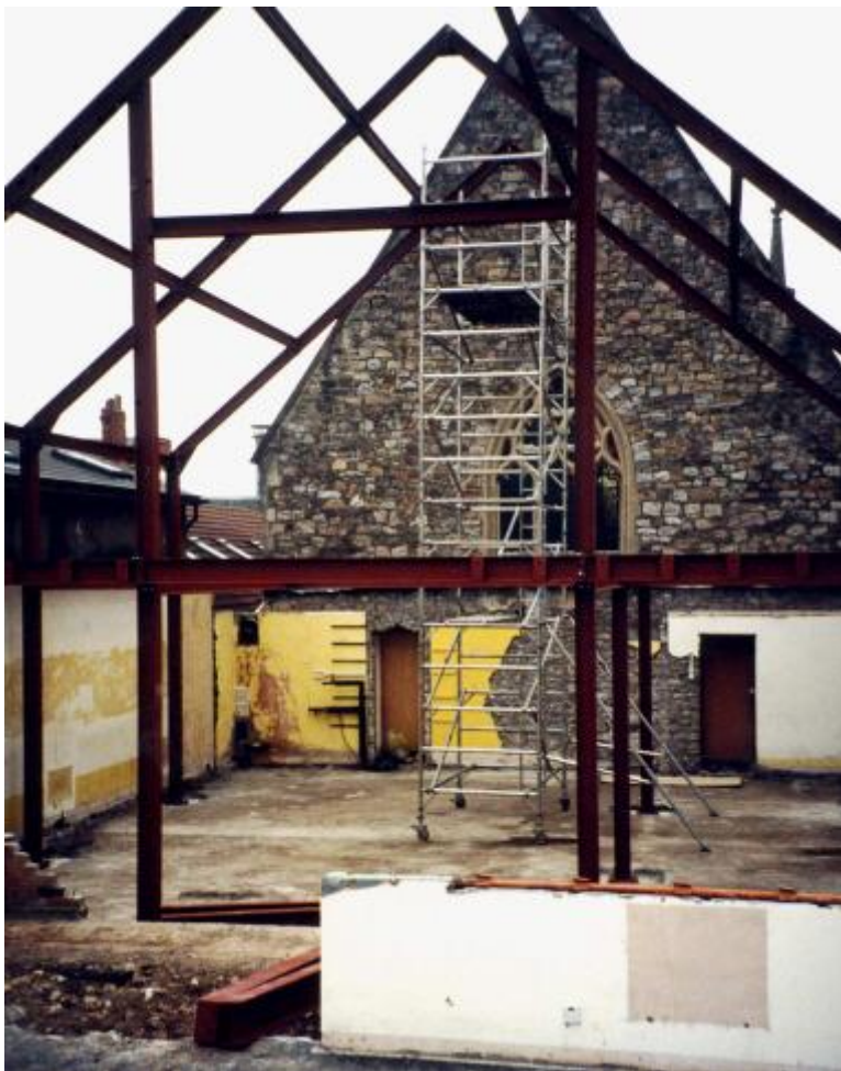
The new building was built on the old foundations. However, it was to be 2 stories high, and therefore a steel frame had to be built on deep foundations.
