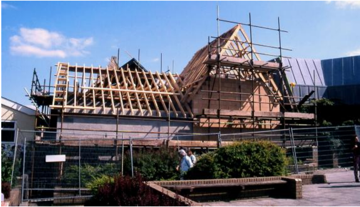
View taken from the back of our premises, almost ready for the tiles
