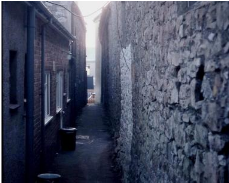
Passageway between Methodist Premises and old third party buildings - note part of the wall is painted white to try to get more light into the kitchen!
